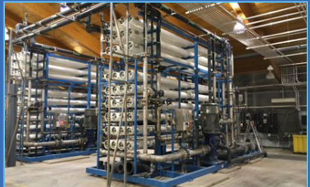
COLORADO RIVER MUNICIPAL WATER DISTRICT RAW WATER PRODUCTION FACILITY
